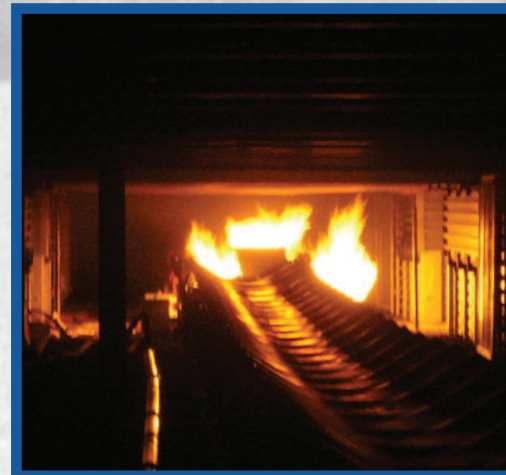
CONVEYOR BELT FIRE
