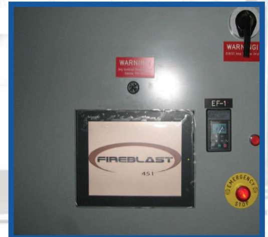
INDUSTRIAL CONTROL RACK
